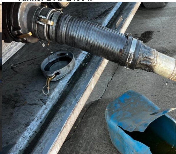
Picture C: Leaking offloading pipe Road Tanker 2 AFQ4304.
