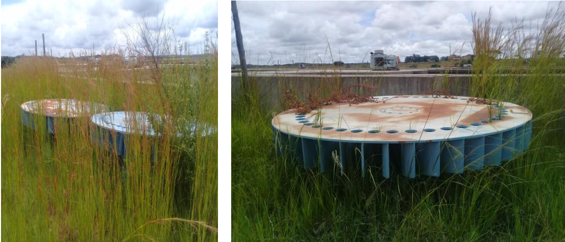
Photo 1- BNR equipment not being maintained
