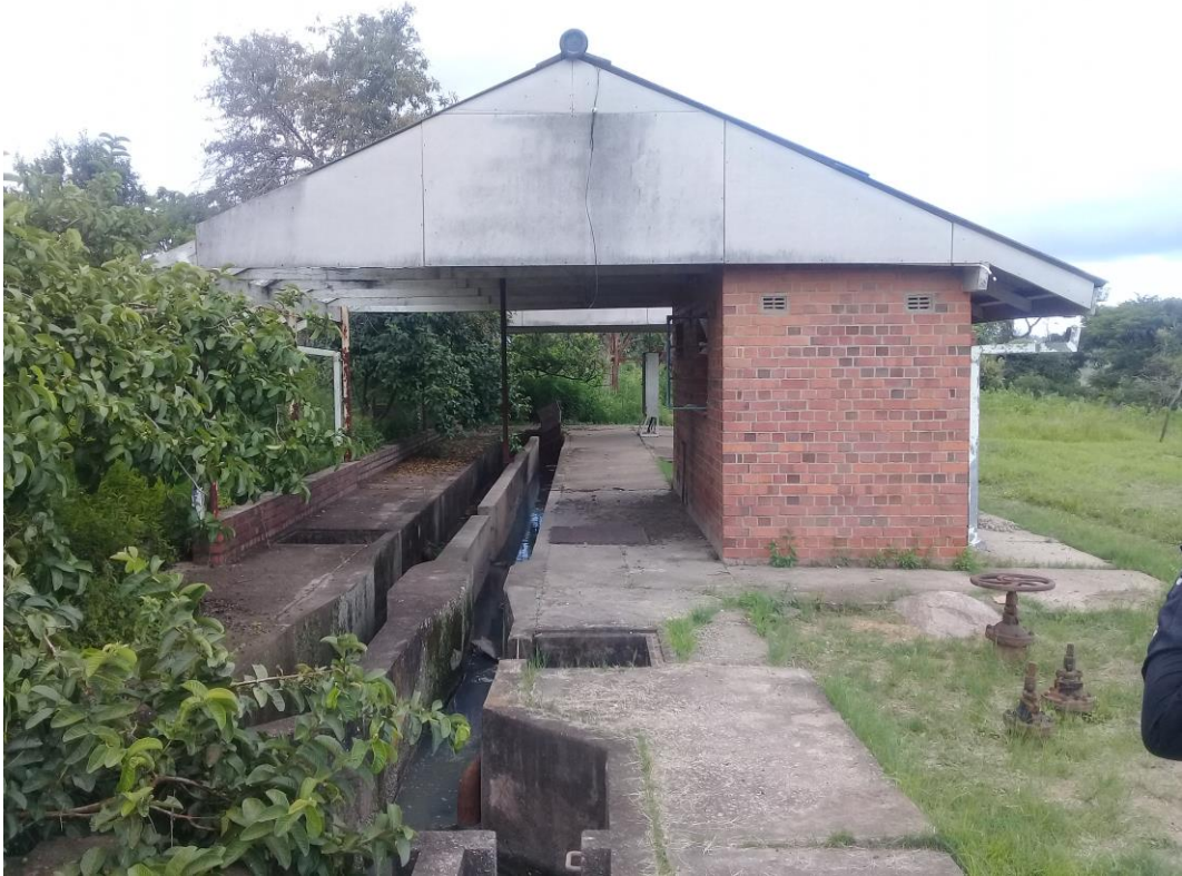
Photo 3- Intake works point not being manned, maintained and the roof falling
