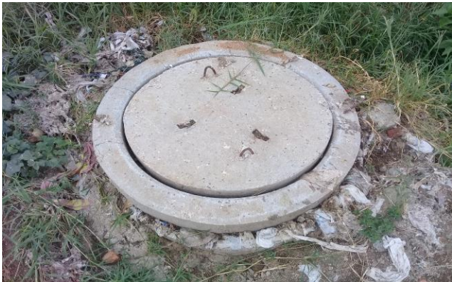
Photo 2- Nketa and Pumula manhole blockages
