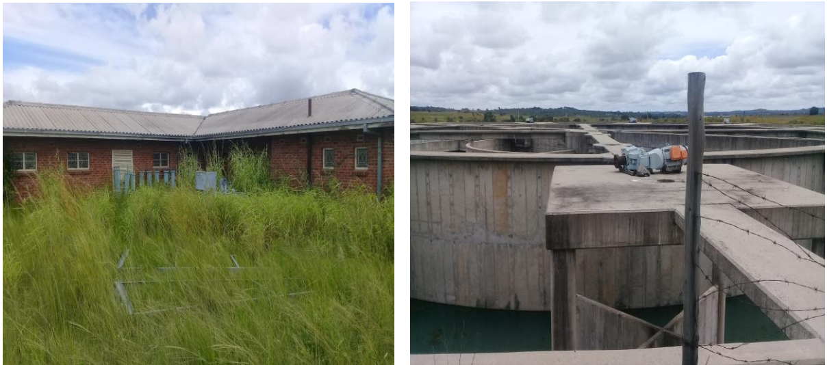
Photo 2- Monitoring offices for the BNR and the BNR not being maintained properly and have not yet been completed
