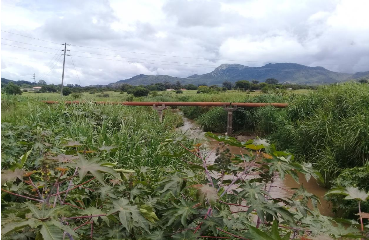
Photo 1- Hobhouse project under repair. Mutare City Council were not using contractors all its project were being done by council.
