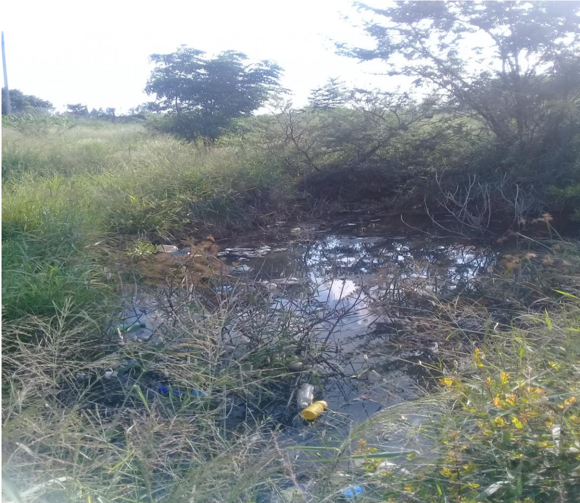
Photo 1- Mucheke Trunk Main Sewer Project still under construction. Beneath the water there are sewer pipes and the area is not being maintained.
